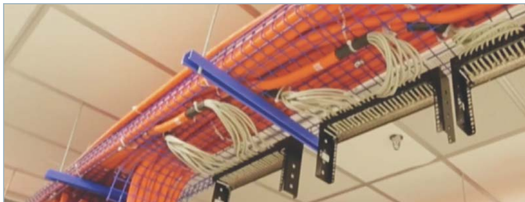
The new Data Center in Nairobi
