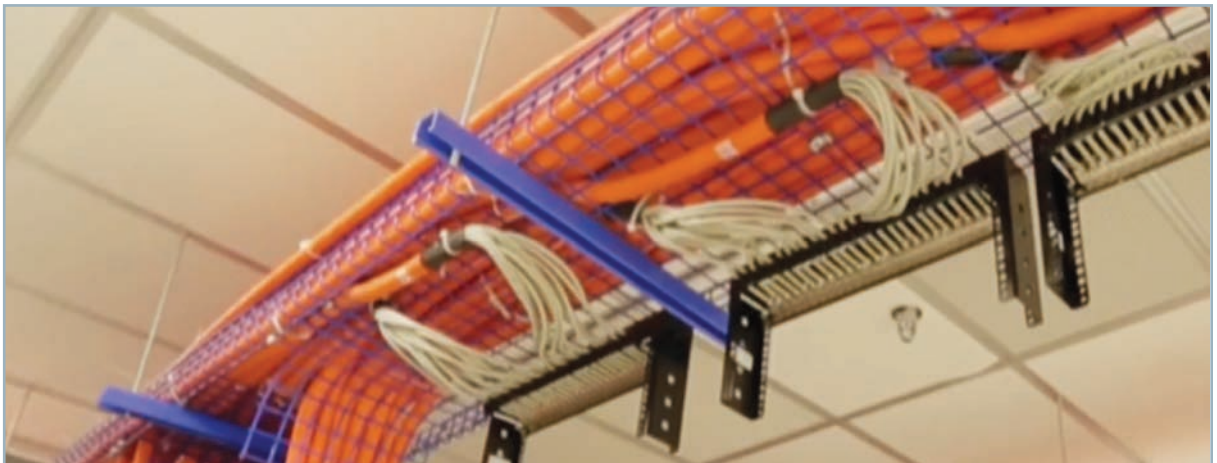
The new Data Center in Nairobi
